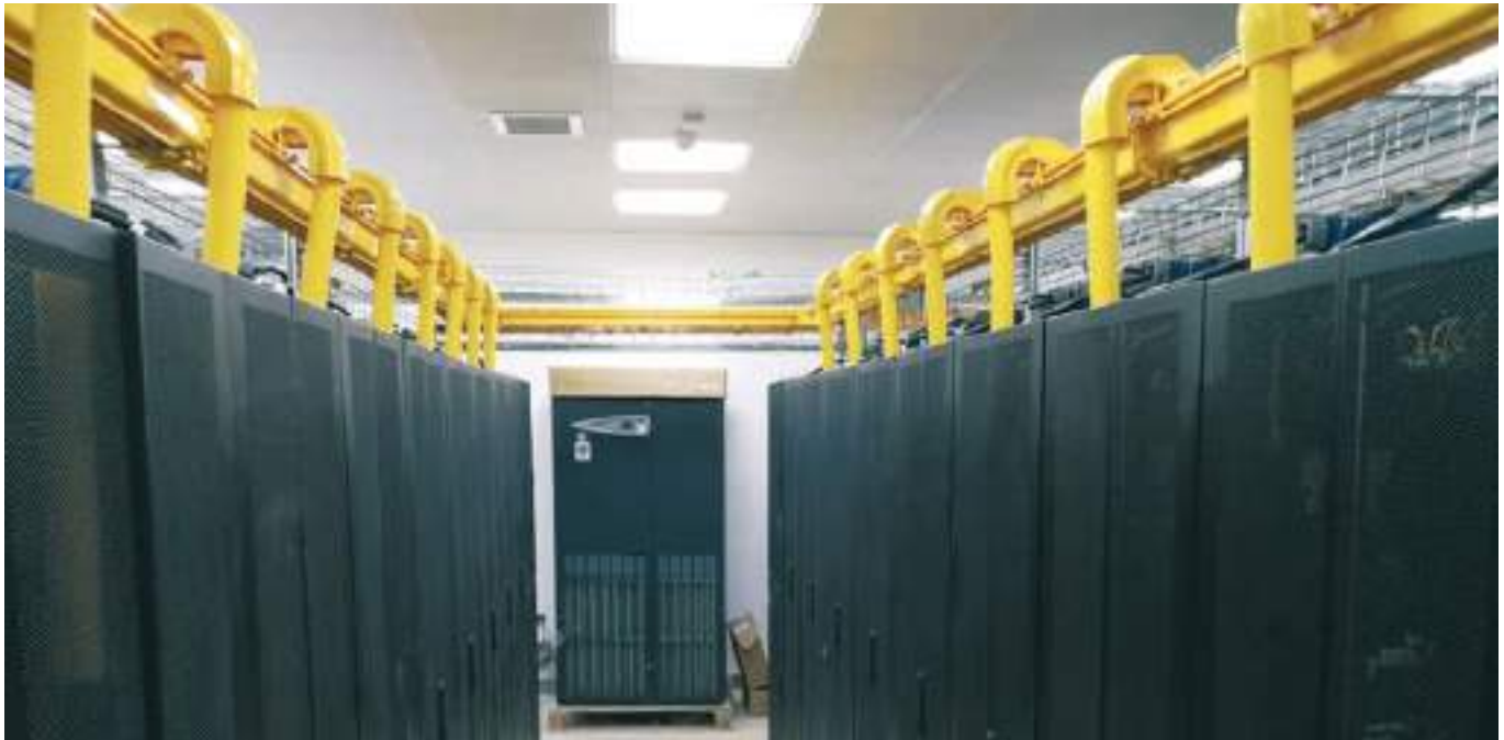
Racks containing servers (data centres)
