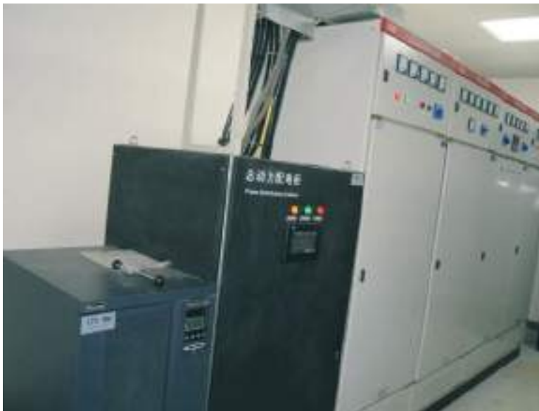
Electric control equipment
