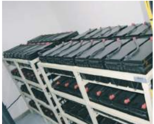
Equipped with 128 batteries to store energy for continuous power supply of all devices in the centre.
